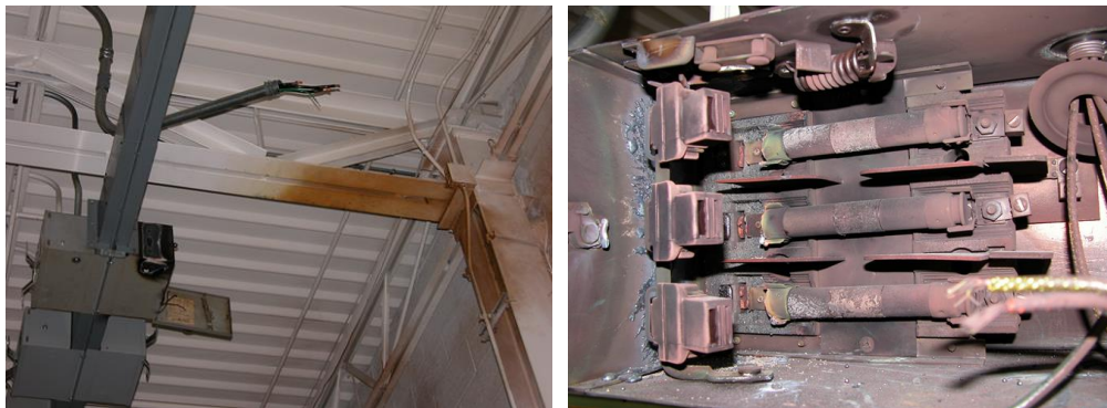
Figure 3-6. Extensive damage to bus plug switch due to an internal arc fault.
