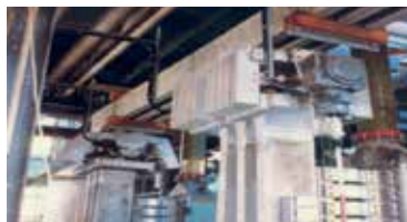
Motor Operated PBD Switch Installed Between Bus Systems, 120kA
