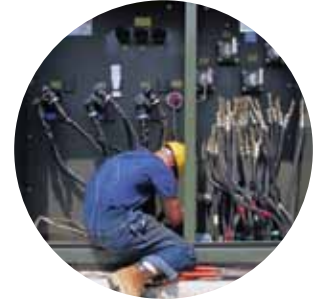
Work on or near energized parts
