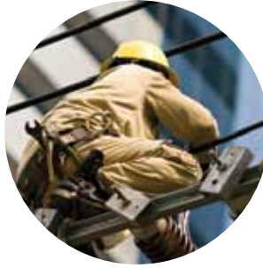
Potential contact with overhead wires
