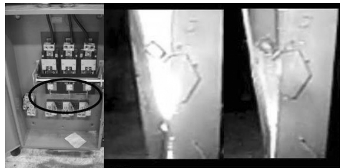
Fig. 9 Latch failure of disconnect with downward plasma flow
