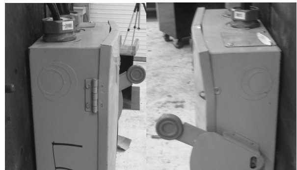
Fig. 7. Damage to the top of door from Test 9 was repaired prior to final test.
