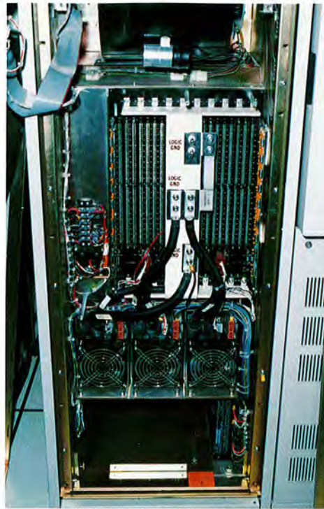
Figure 1. A cabinet-mounted card cage receives its power from the two-conductor, I-shaped bus seen at the center of the cabinet. (Eldre)
